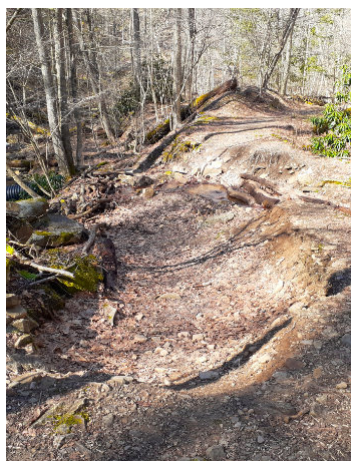
Washed out bank and culvert
